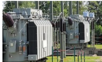
Electrical Power Distribution
